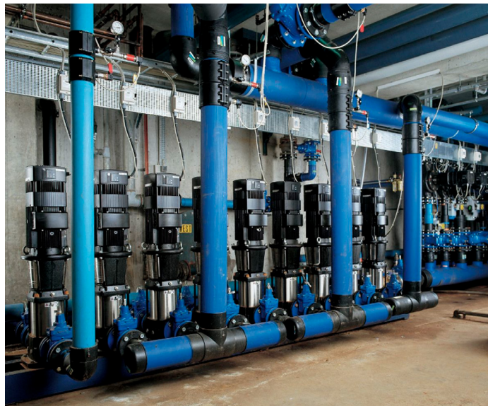
A row of Grundfos CRE E-pumps for circulation of cooling water in a machine tool factory
