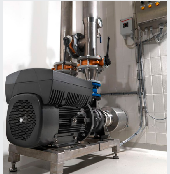
An NBE E-pump at the ARLA Foods Arinco dairy in Denmark
