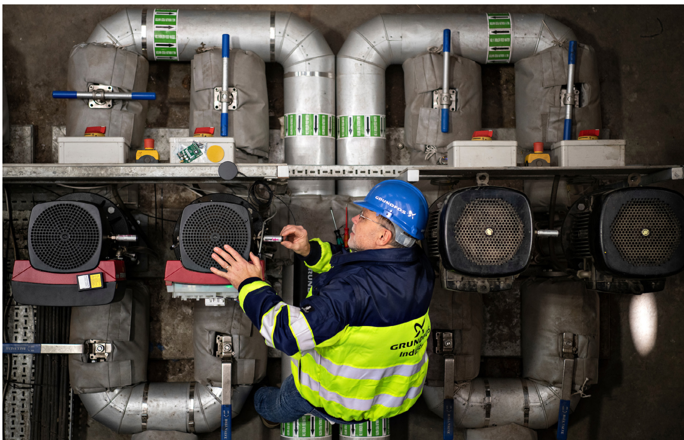
Grundfos Senior Application Manager Michael Rasmussen at one of the new CRE pumps for the boiler feed level control at William Grant & Sons' Girvan Distillery in Scotland.
